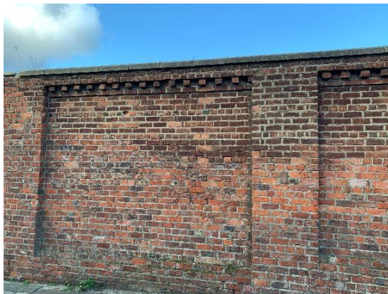
Photograph 11: Wall Section 4, top section of wall has been re-built with brickwork to try and match original brick.
