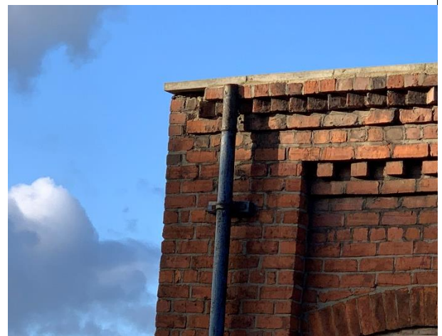
Photograph 8: Wall Section 3, loose / missing mortar to coping.
