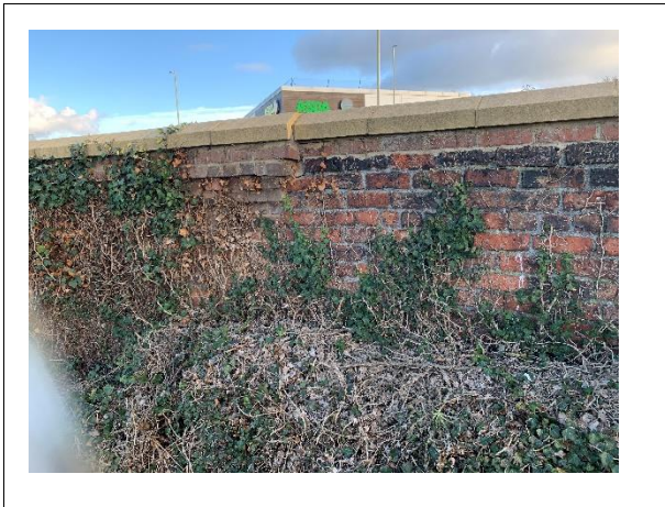
Photograph 17: Wall Section 4&5 junction with, vegetation growing up the rear face.
