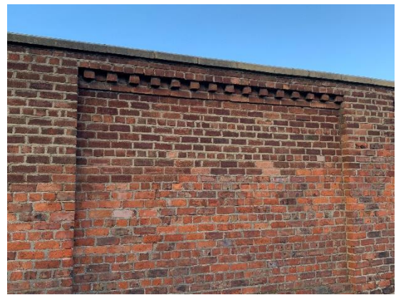
Photograph 12: Wall Section 4, top section of wall has been re-built with brickwork to try and match the original brick.
