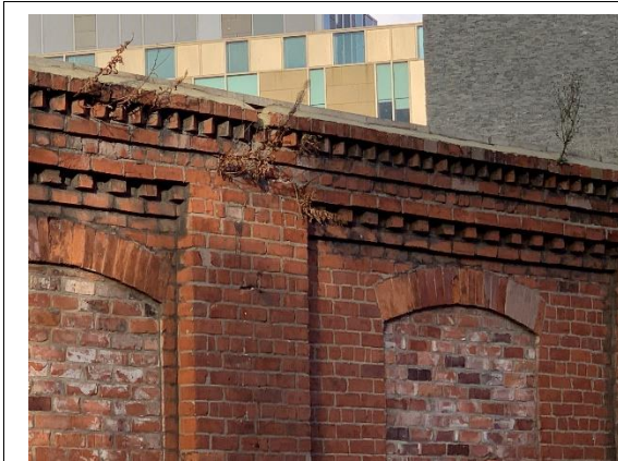
Photograph 9: Wall Section 3, vegetation growing for the old gutter position at the wall head.
