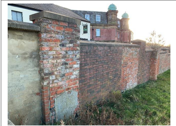
Photograph 25: Wall Section 2, rear face has been repaired and rebuilt in local sections. Joint not bonding through
