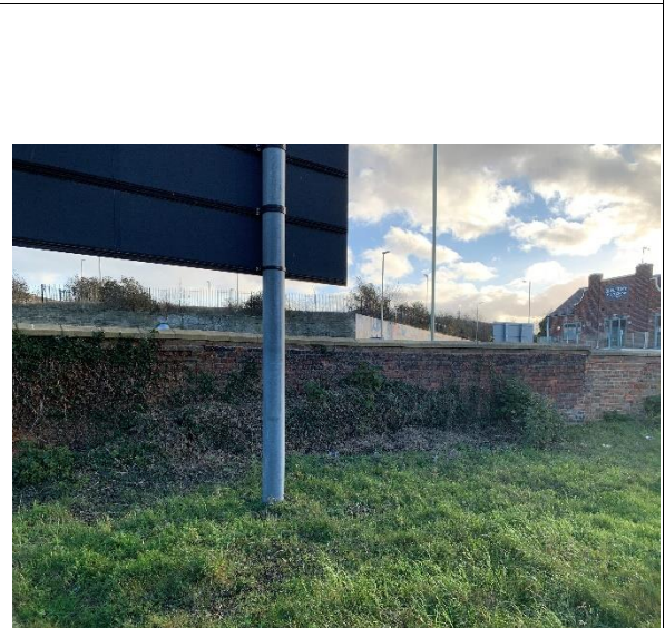
Photograph 16: Wall Section 4 & 5, vegetation growth to rear of wall.
