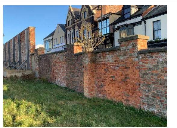
Photograph 26: Wall Section 2, vegetation growth and local rebuild.
