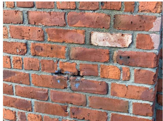
Photograph 10: Wall Section 3, mortar loss to joint.
